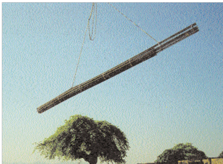
A Bamtec reinforcement mat on the hook. The structural steel is delivered to the place of installation at the construction site just-in-time.
