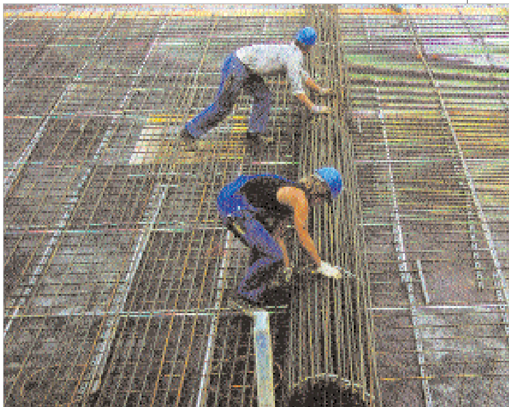
Depending on the structural analysis, several layers of Bamtec reinforcement mats can be placed on top of each other.
